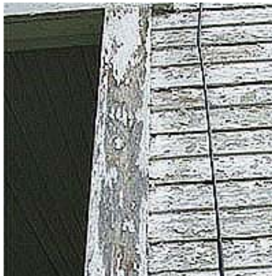
Paint Peeling on a House
